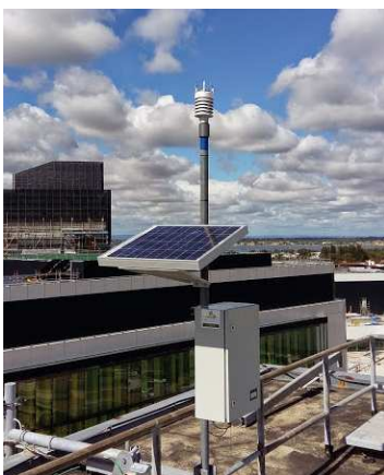
Vaisala Weather Station – Temp, RH, Wind Speed and Direction, Rain, Baro Pressure
